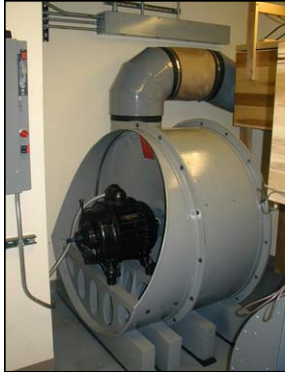
newly-installed Spencer blower for Orchestra Hall, Chicago
